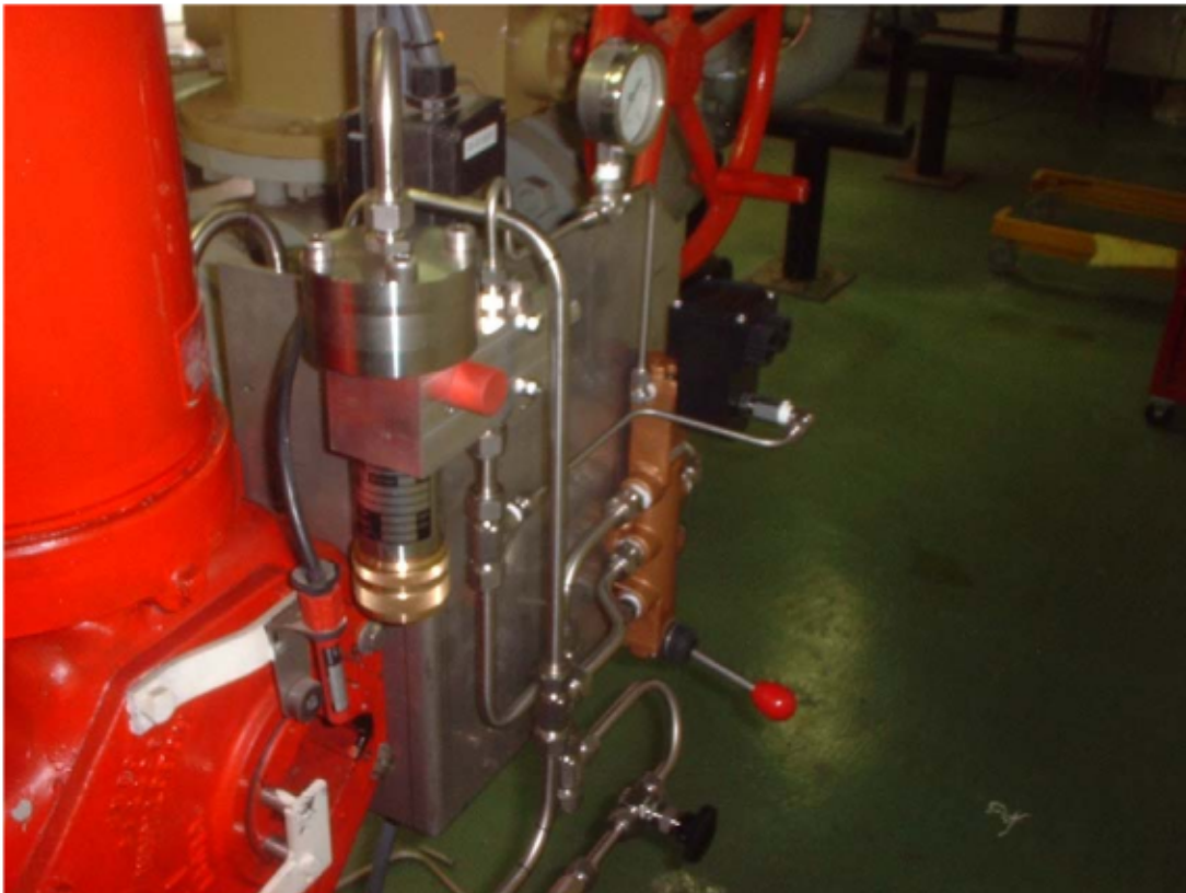
Fig 8.2 Control Pilot HON CP52 in Remote Control Loop as Shut-off Override
